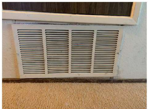
HVAC Filter Location
