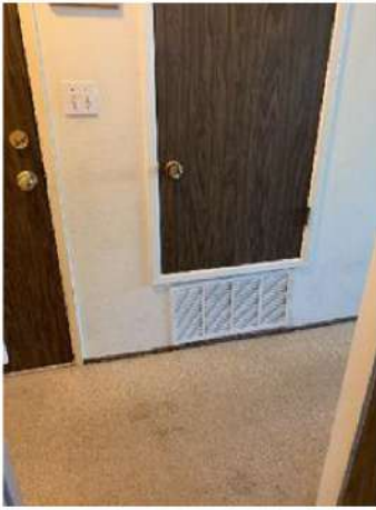
HVAC Filter Location
