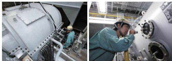
Inspections surrounding a steam turbine
