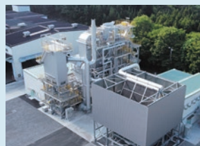
Fukushima Hirata Biomass Power Unit No. 1
