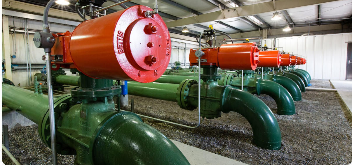
Northwest Pipeline located in Sumas, Washington.
