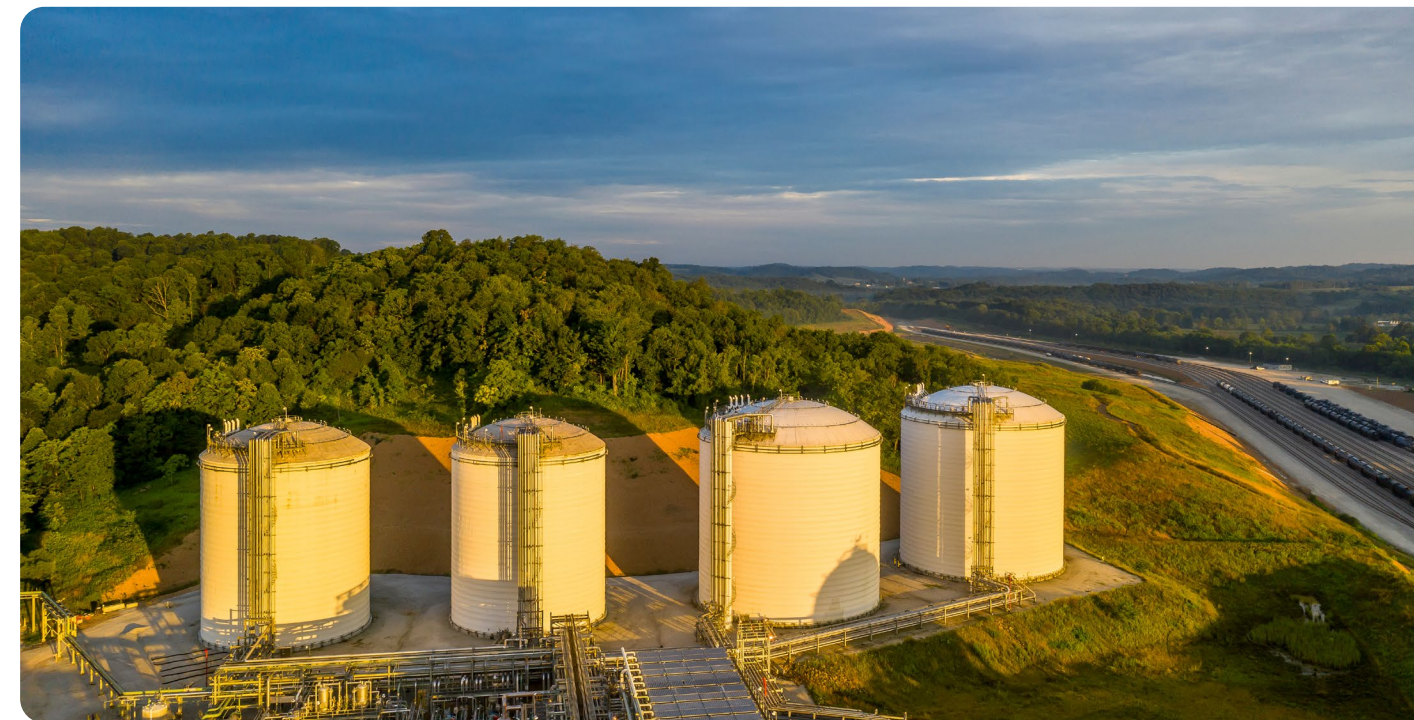
Harrison Hub Fractionation Plant in Scio, Ohio.
