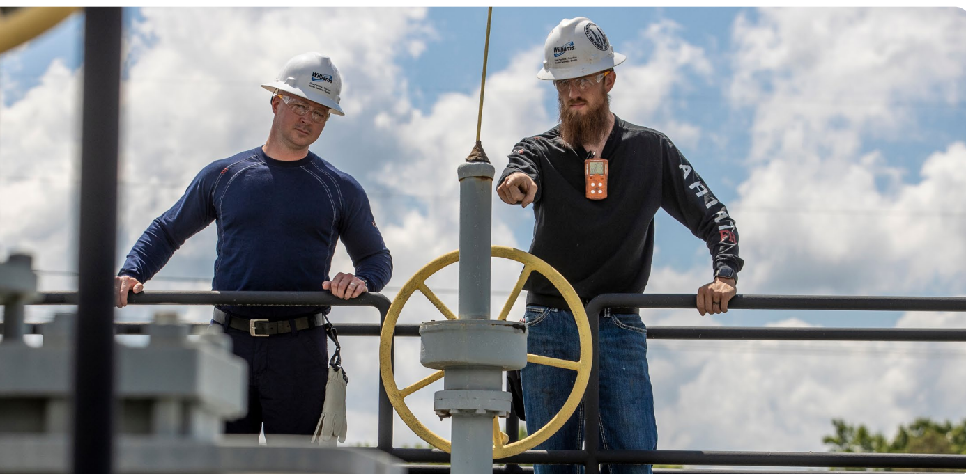
Jeff King, Senior Operations Manager, and Michael Watkins, Training Specialist at the Transco Pipeline Station 145 in North Carolina.
