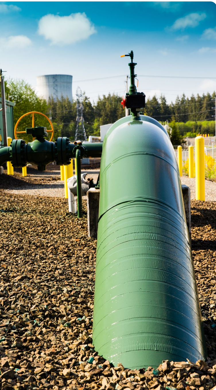
Grays Harbor Metering Station in Aberdeen, Washington.
