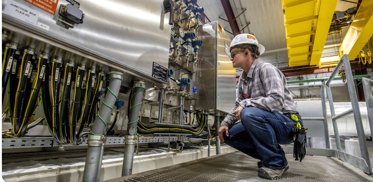
Katie Durcik, Maintenance Coordinator at the Transco Pipeline Station 610 in Millerville, Pennsylvania.
