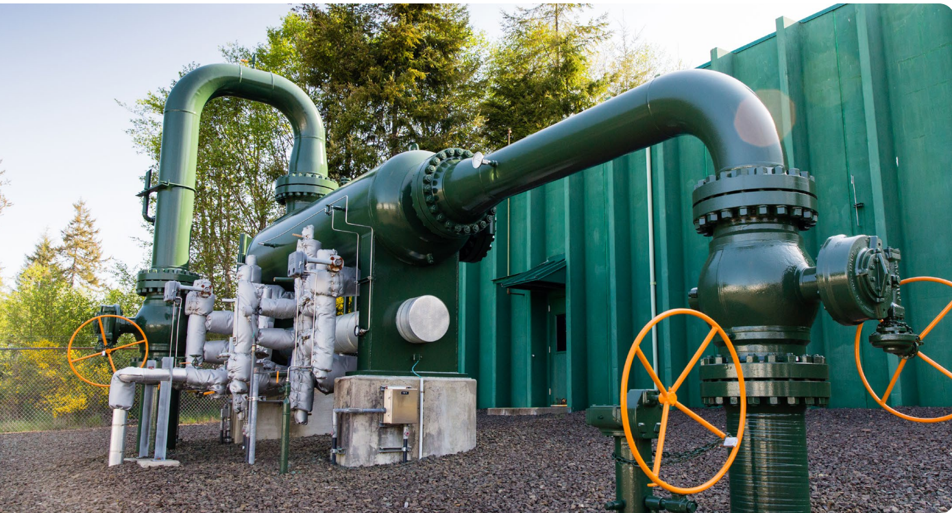
Grays Harbor Metering Station in Aberdeen, Washington.
