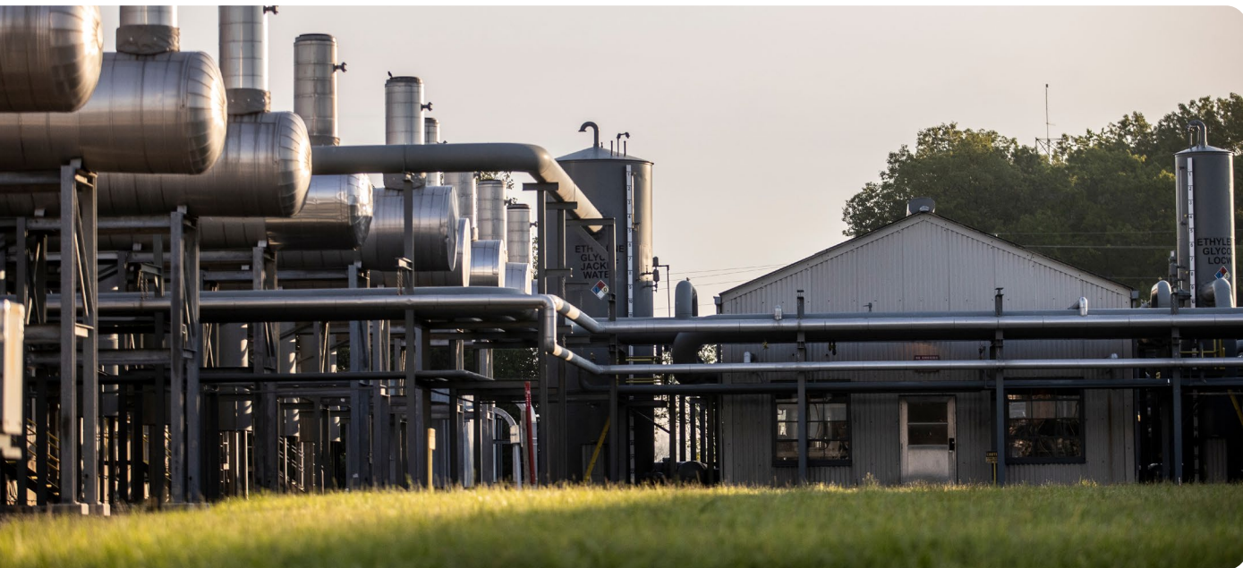
Transco Station 185 in Manassas, Virginia.
