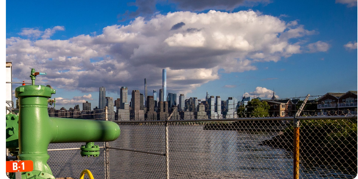
72nd Street Valve Site in North Bergen, New Jersey.
