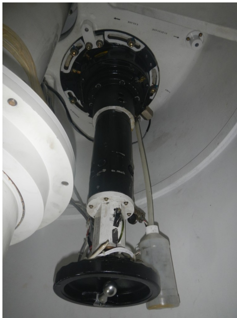
Motor attached to the gearbox. This is inside the pedestal.
