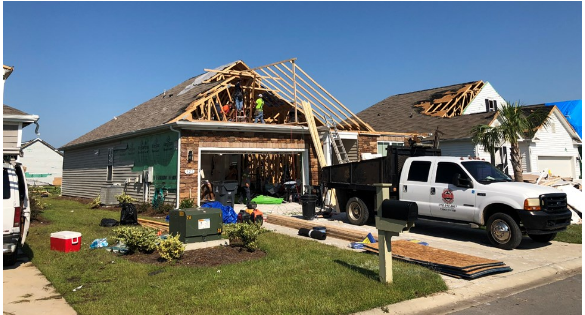
NWS meteorologists conducting a storm survey took this photo of damage to homes in Carolina Shores, Brunswick County, NC, after the early morning tornado of September 5, 2019.
