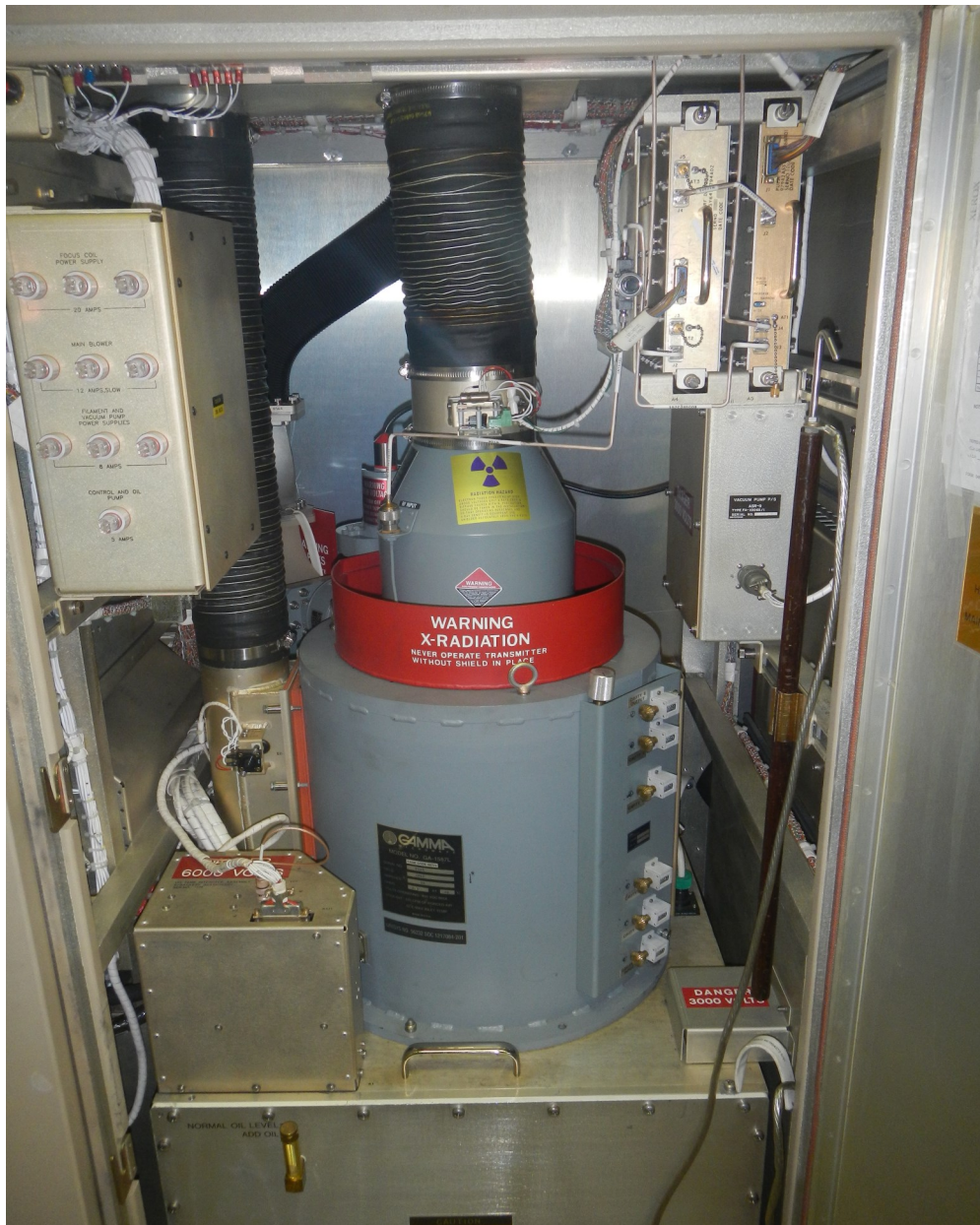
The Klystron, the main power amplifier of the NEXRAD transmitter.
