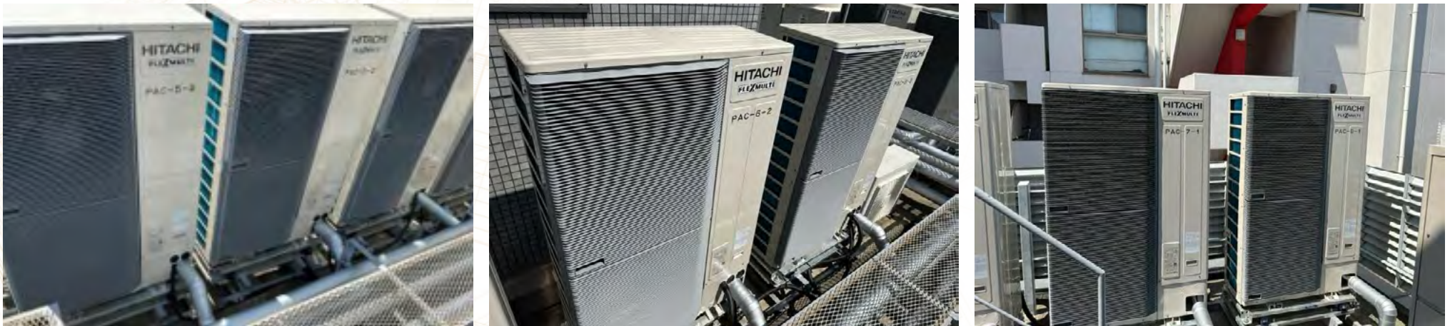
REPLACEMENT TO HIGH ENERGY EFFICIENT AIR-CONDITIONING SYSTEM AT ITACHIBORI SQUARE, OSAKA, JAPAN
