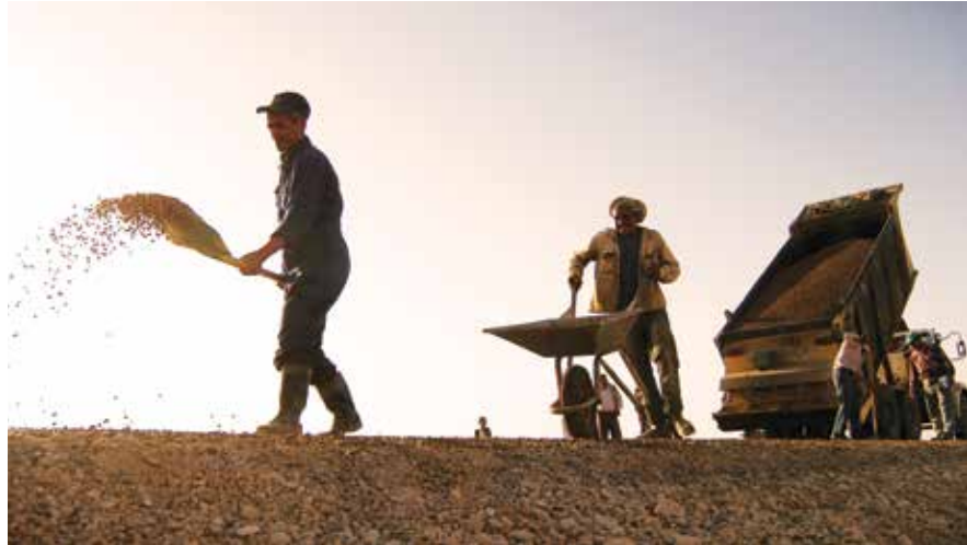
Many millions of dollars flow into road-building contracts in Afghanistan. (USAID photo)
