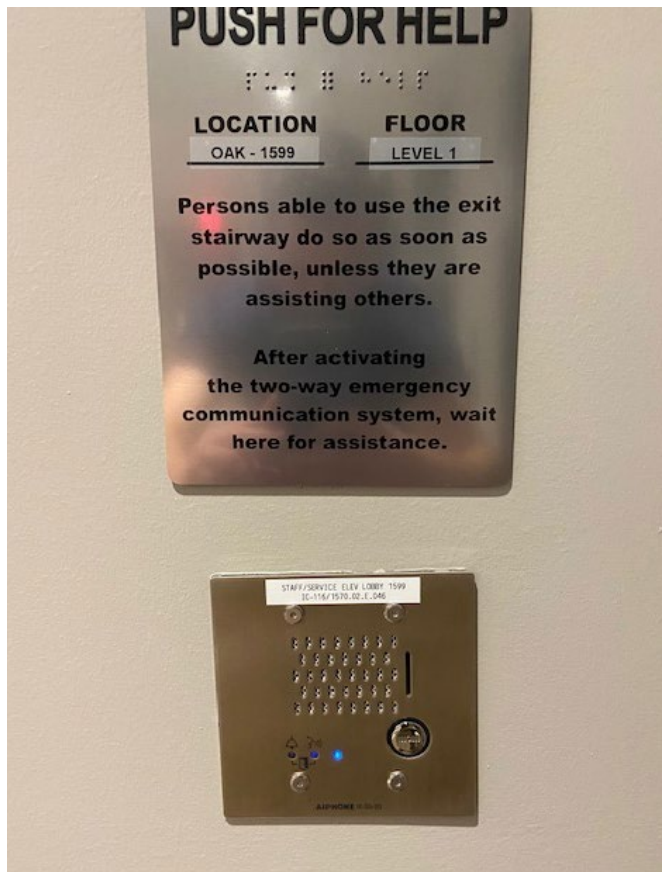
Compact IP Audio Door Stations (IX-SS-2G) were installed in medical and surgical rooms, waiting rooms, intensive care units (ICUs), and newborn intensive care units (NICUs).
