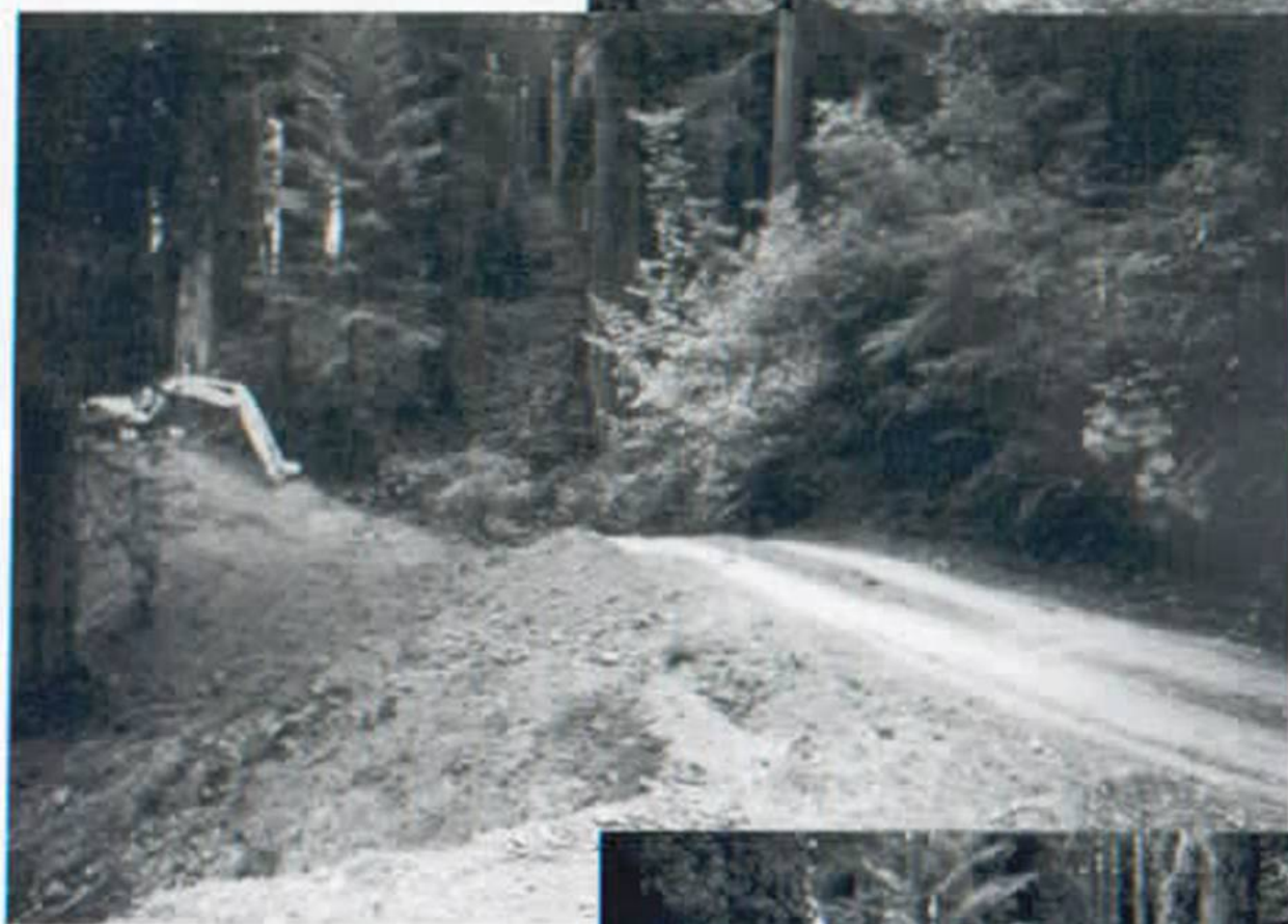
DURING Ah Pah Road During restoration — excavation of road fill down to original stream channel.
