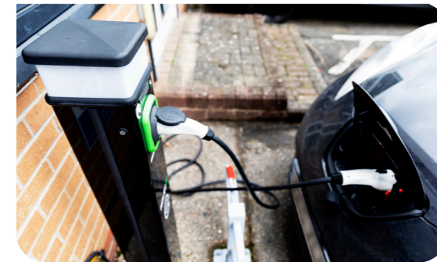
NSSLGlobal free electric charging point
