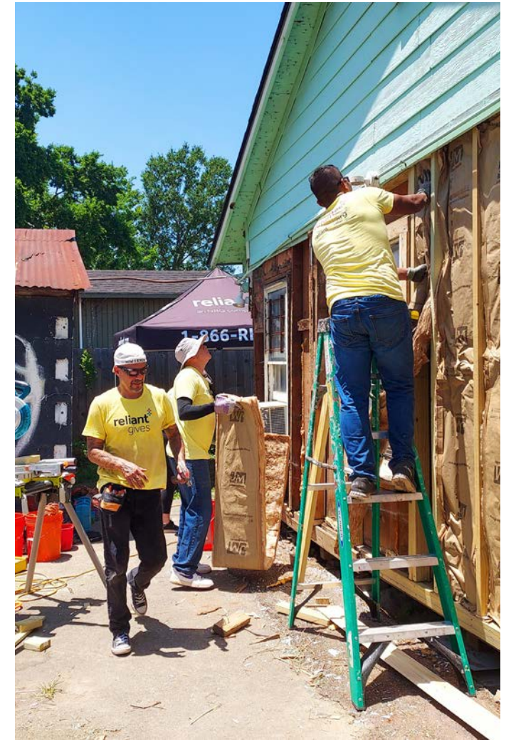
Volunteers helped to repair a home built in 1949 whose owner had lived there for 33 years. The effort helped to make the home comfortable to live in for many more years to come.
