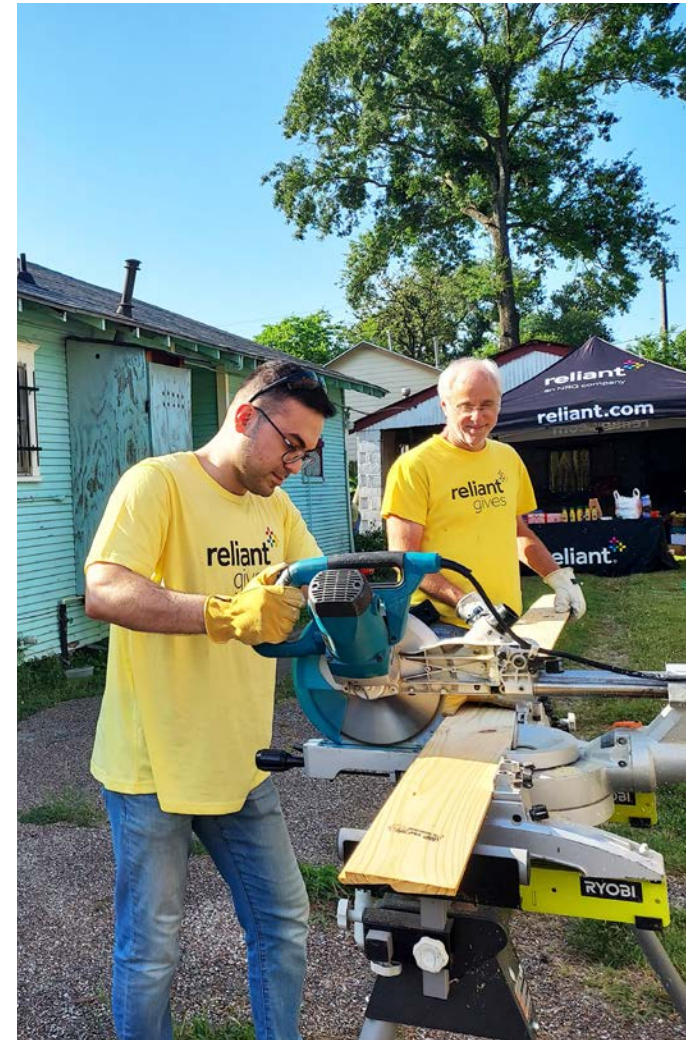
Reliant volunteers helped build a wheelchair ramp for a 90-year-old U.S. Army veteran, allowing him to safely enter and leave his Houston home and improving his quality of life.
