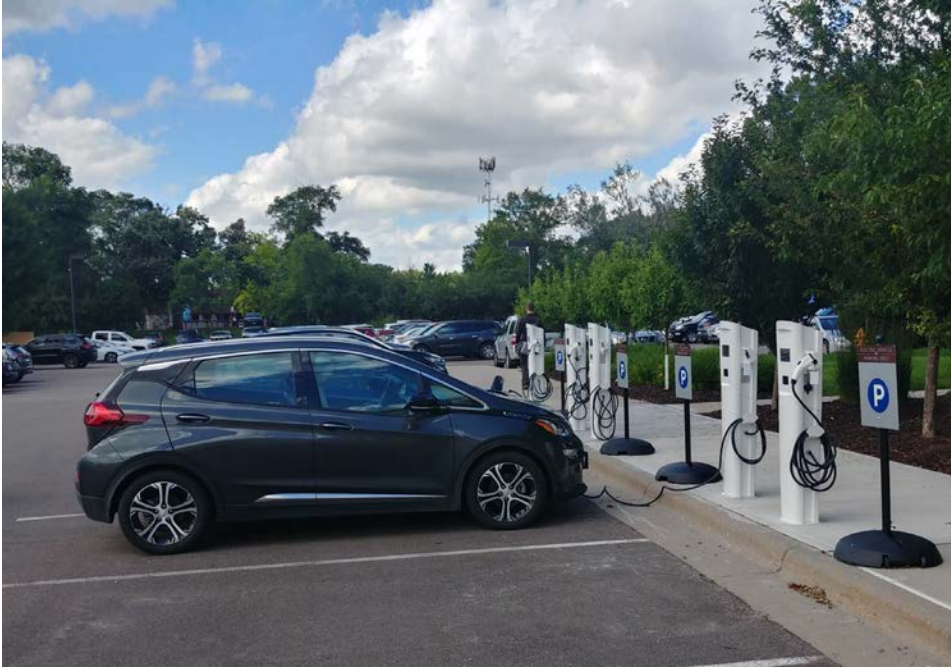
Workplace charging in surface parking lot at Mortenson Construction headquarters. Photo credit: Brian Ross
