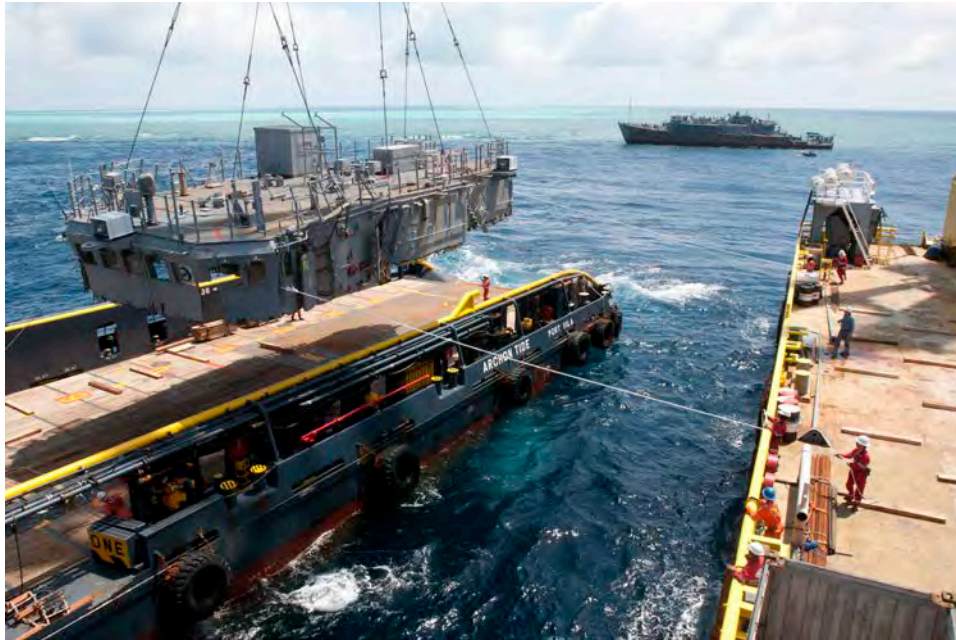
Figure 5-12. 02 level being transferred from JASCON 25 to Archon Tide for further transfer to barge S-7000. Note GUARDIAN in background with 01 level remaining.
