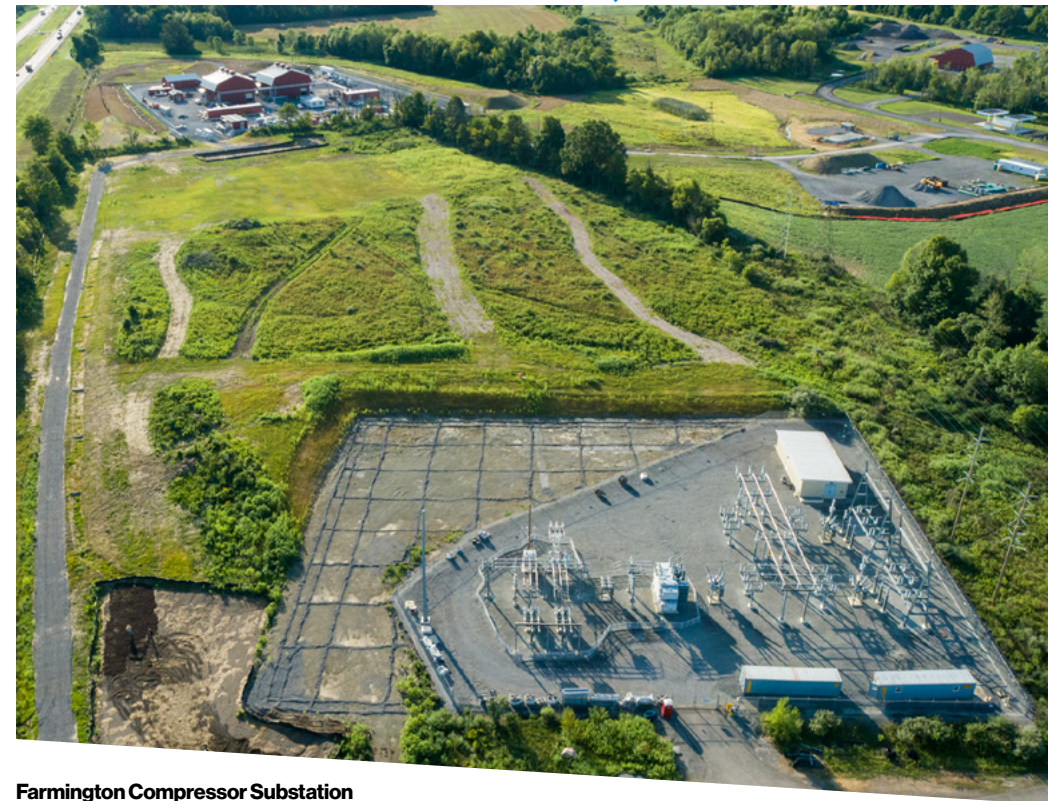
Farmington Compressor Substation Farmington, New York
