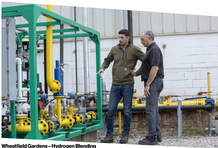
Wheatfield Gardens – Hydrogen Blending Demonstration Project at Greenhouse Facility
