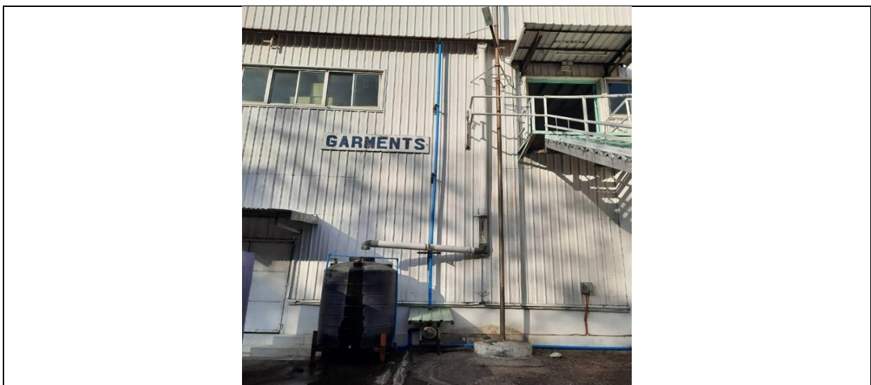
Collecting the water sprayed on the roof for cooling and pump it back to the roof for reuse
