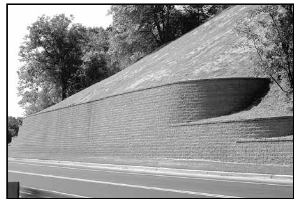
Return walls create a terraced appearance instead of a series of short steps at the top of the wall.
