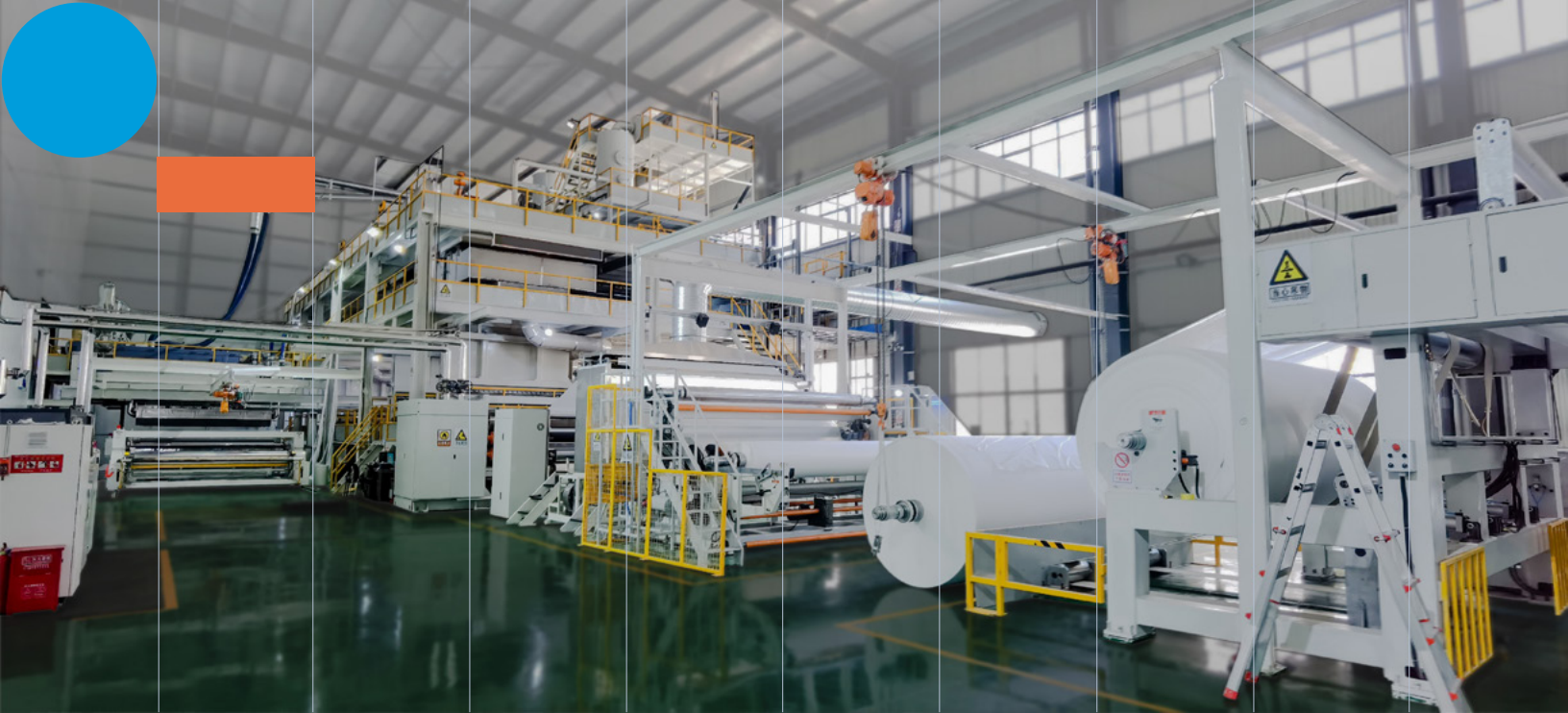
Spunmelt production line. Credit: Suntech Textile Machinery
