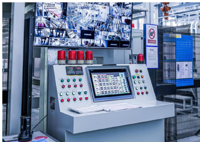
Nonwovens production controls. Credit: Guangdong Yizhou Advanced Materials
