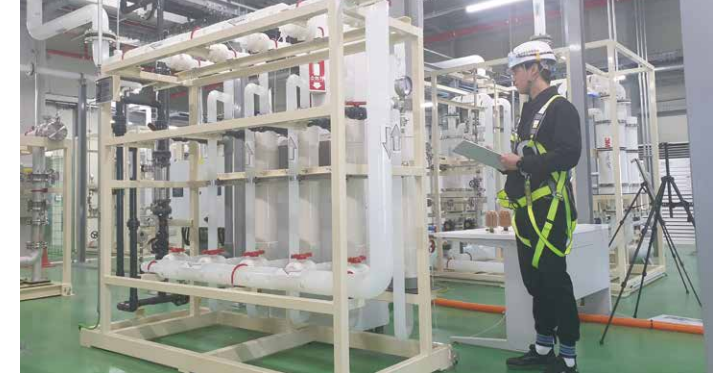
Inside the Ultrapure Water Validation Plant
