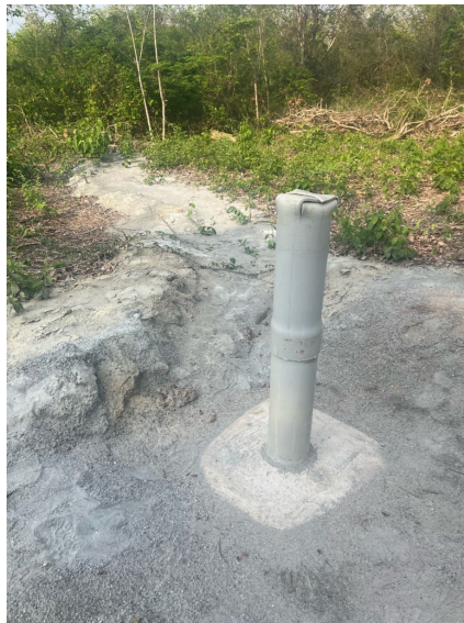
Picture 1: Sealed well in Portoncito, San José de Chiquitos drilled by the Contractor according to the community.
