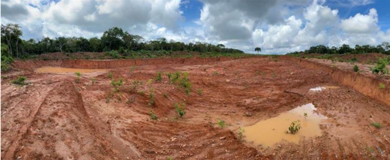
Picture 3: A site where the Cuarrió, San Miguel community claim the Contractor had removed topsoil to use in the road construction.
