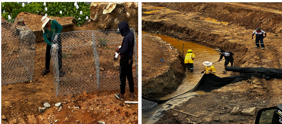
Pictures 10 and 11: Workers without appropriate PPE, observed by the Panel, adjacent to the road corridor.
