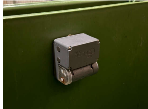
Smart bin sensor installed inside the litter bin
