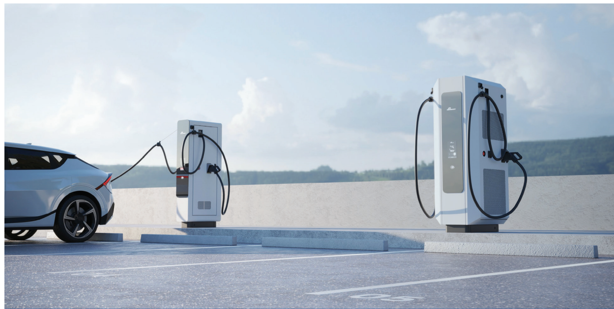
To help reduce our greenhouse gas emissions, HWC is committed to installing electric vehicle charging stations throughout our footprint.
