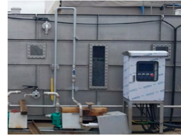
Reuse of runoff groundwater from the construction site (Geomdan Incheon Subway Line 1)
