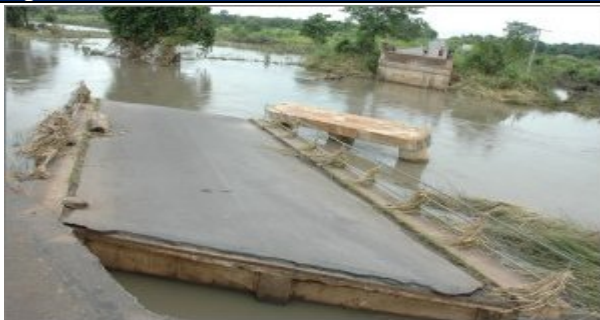
2008 Amakpape National1 bridge destroyed by heavy rains
