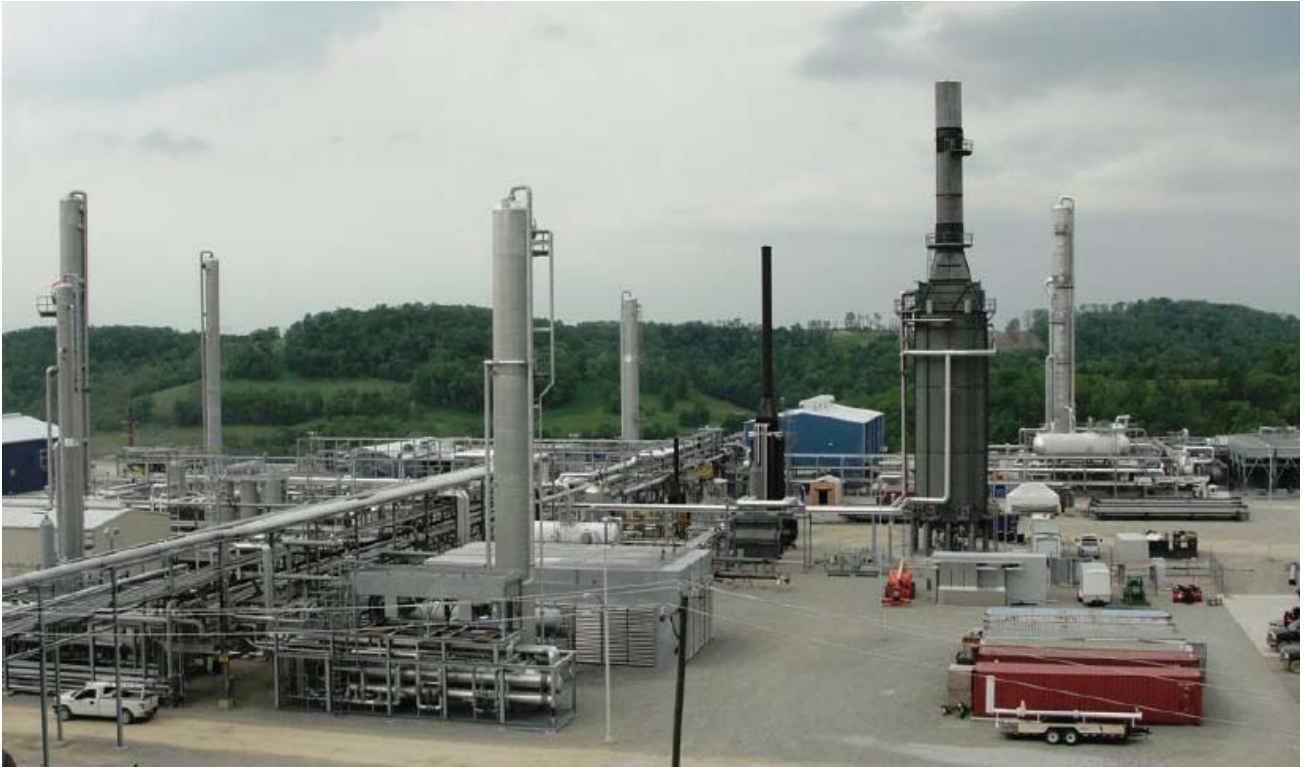
Figure B8.9 Gas processing and cryogenic plant, Pennsylvania 16
