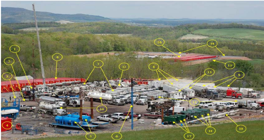
Figure B8.2 A US shale gas site during a single hydraulic fracturing operation 6
