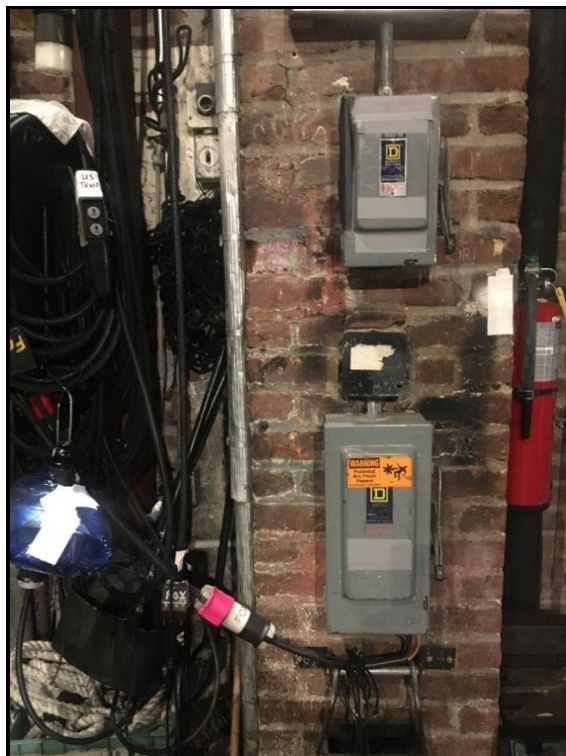
POWER DISCONNECT UP STAGE RIGHT (USR)
