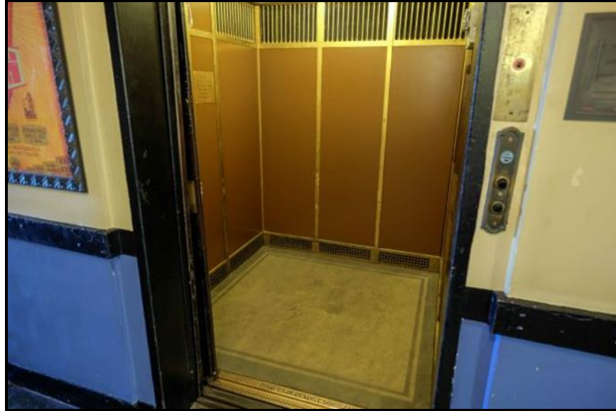
BACKSTAGE ELEVATOR FOR DRESSING TOWER USAGE
