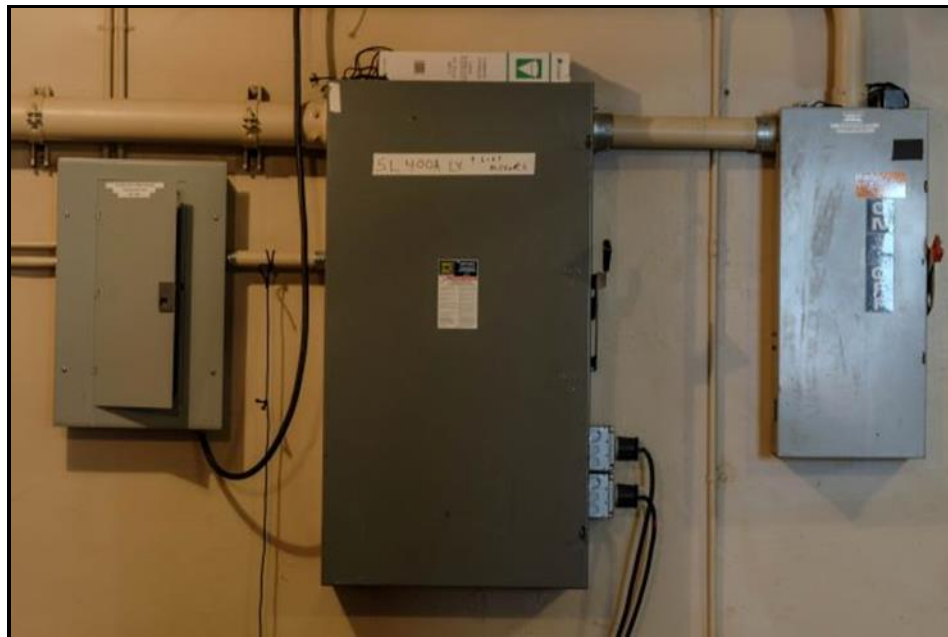
POWER STAGE LEFT PROP ROOM
