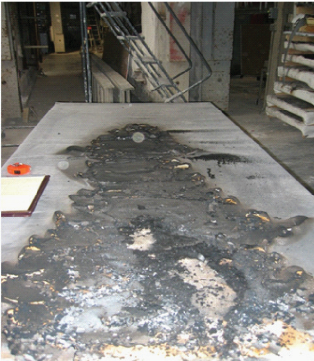
Photo 4 – FR rated EPDM over Dens Deck, very irregular flame pattern
