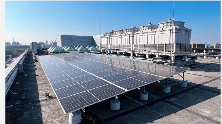
Newly installed rooftop solar panels at our fabrication site in Shanghai
