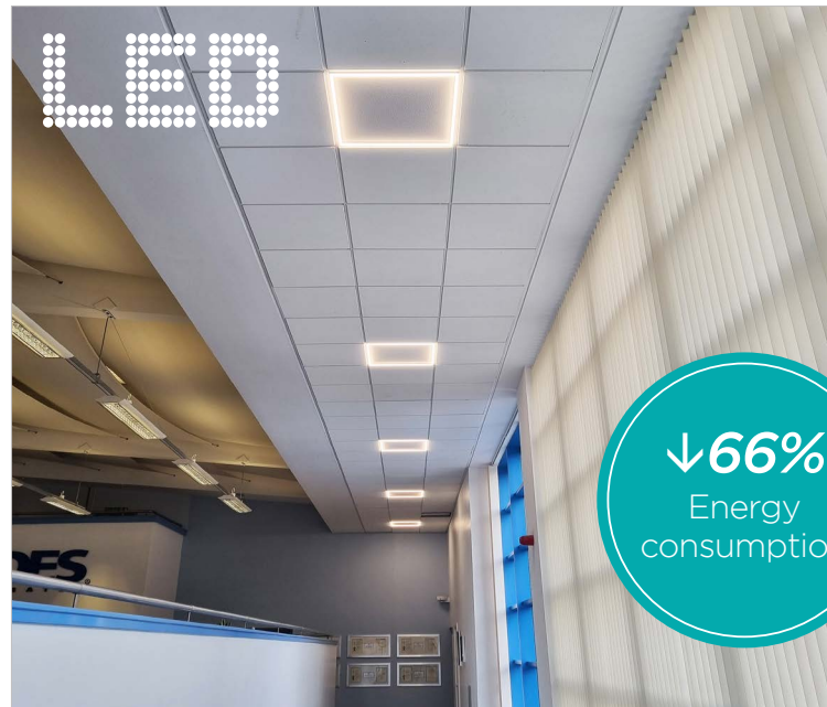
LED lighting at our Oldham (UK) facility
