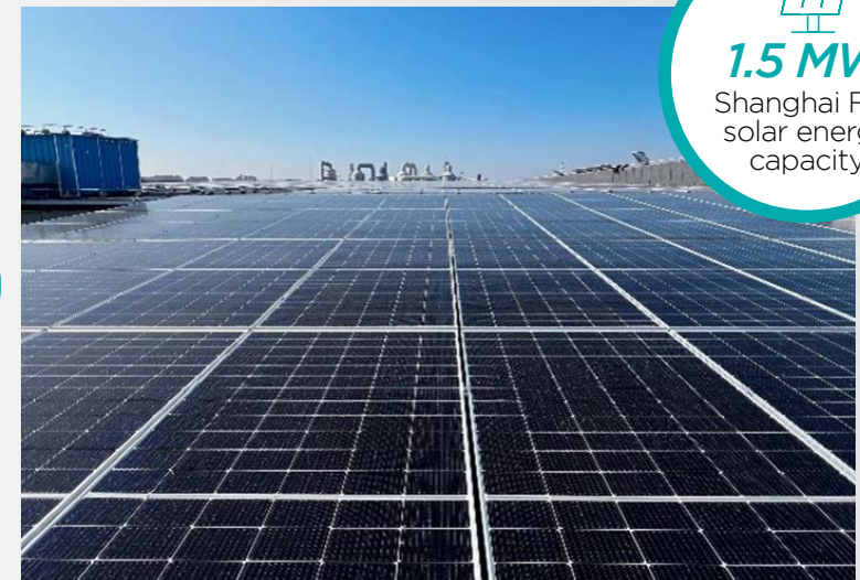
Newly installed rooftop solar panels at our fabrication site in Shanghai
