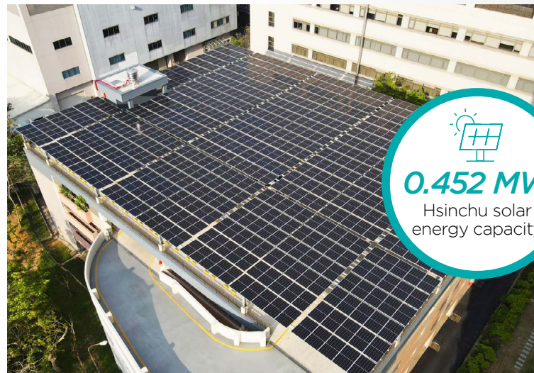
Newly installed rooftop solar panels at our fabrication site in Hsinchu
