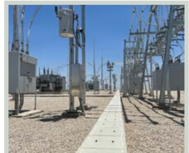
Substation: Part of Coterra’s Electrical System
