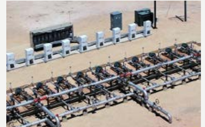
Booster Station: Part of Coterra’s engineered system for water reuse
