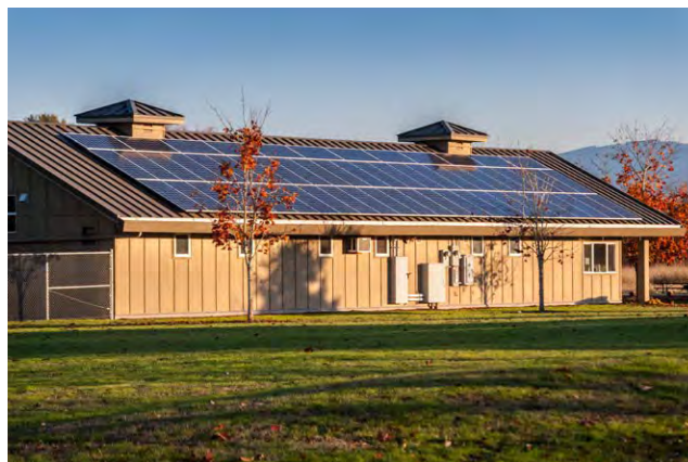
Solar panels on roof of North Utility Building at Marymoor Park, WA.
