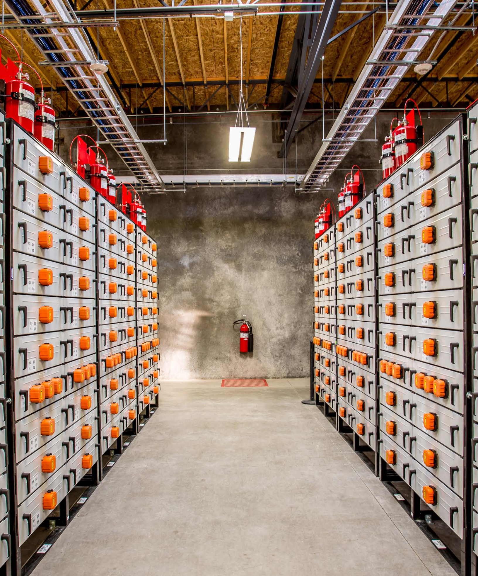
Portland General Electric's Salem Smart Power Center includes a large-scale energy storage system. Portland General Electric
