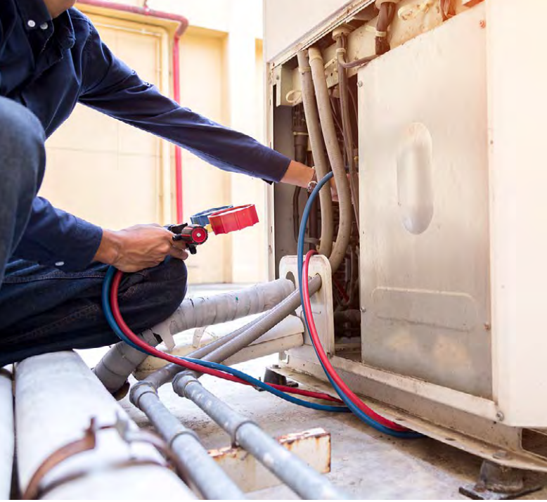
Technician measuring air conditioning equipment.
