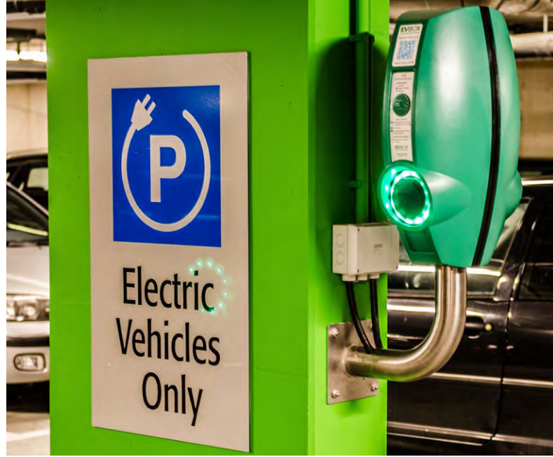
EV charging station. stanvpetersen
