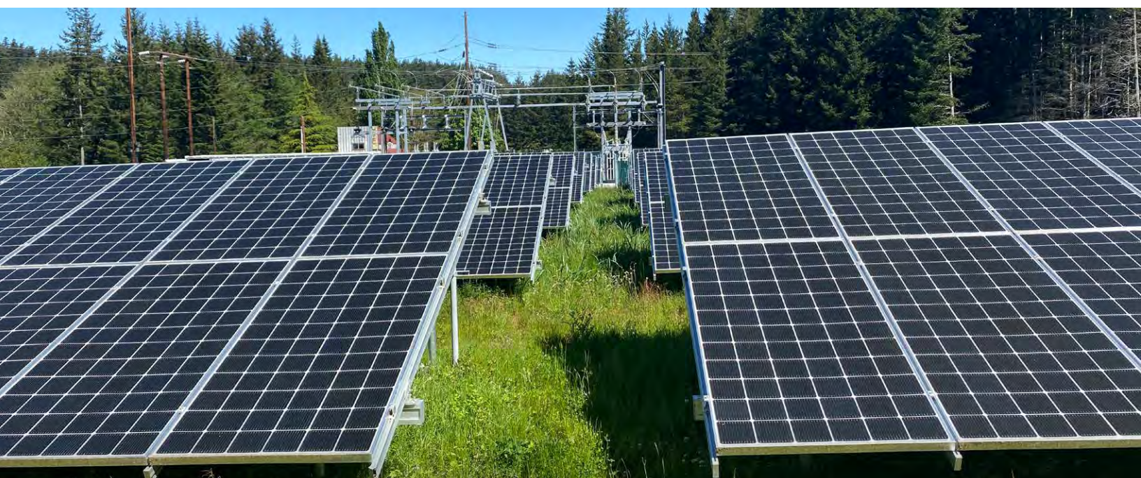
Solar installation at the Decatur Island Community Solar Project. Orcas Power & Light Cooperative
