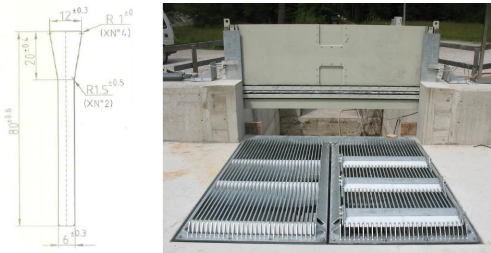
Figure 3: Bar profile and sizes [mm] (left) and screen + sluice gate seen from the head water (right) - gate raised and without the overflow profile - see Figure 4 for the overflow profile
