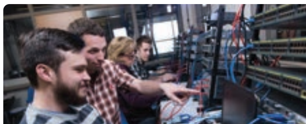
Students working with the instructor using Cisco networking hardware in one of SMCC's labs.
