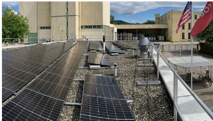
Solar array on roof in Rheinfelden, Germany
