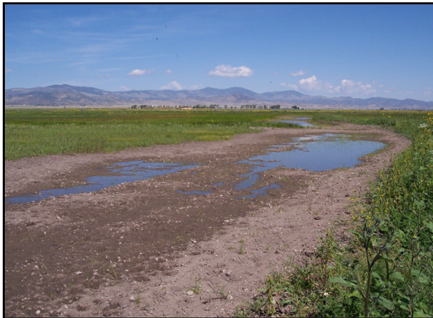
CWP wetland project incorporating rest rotation grazing and construction of contour levees and water control structures on private land; San Luis Valley Wetland Focus Area.
