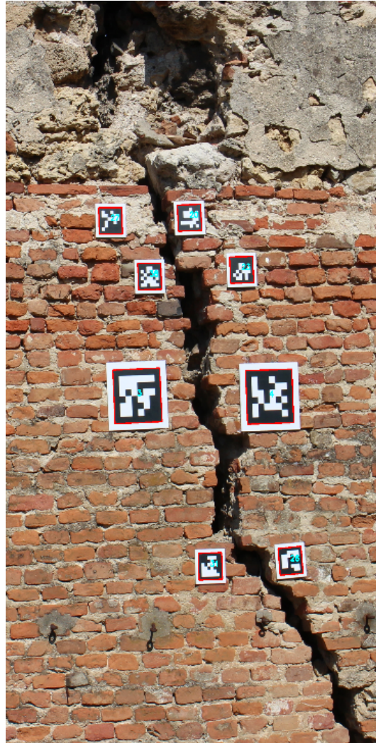
Fig. 2. ArUco fiducial markers have been placed along the crack in the most critical points. The markers are correctly detected and identified.
