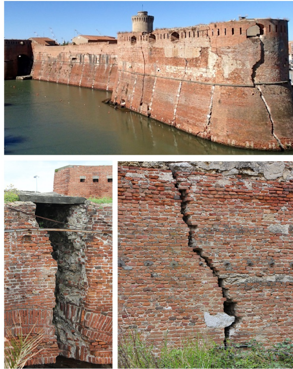
Fig. 1. Evident structural defects in the walls of the ancient fortress, in the area named Bastione della Capitana (Fortezza Vecchia, Livorno, Tuscany, Italy).
