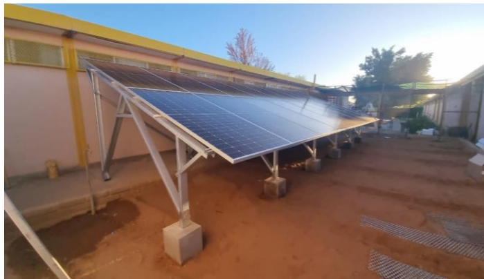
PV system installed at a school
