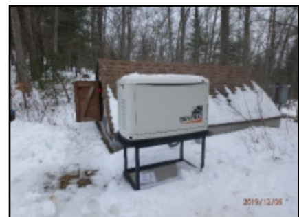
Wilmington Ridge Emergency Generator Connecticut DWSRF 2020 Annual Report
