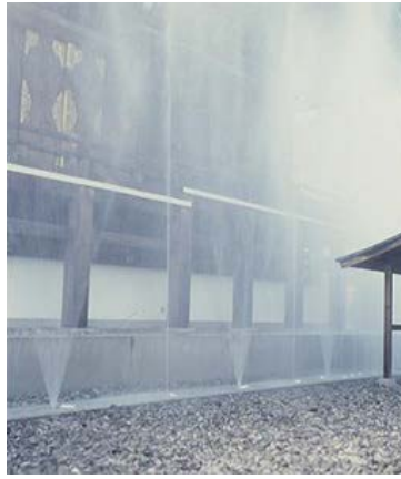
Drenchers which prevent a fire from spreading
