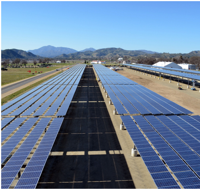
Solar panel arrays form a canopy at a construction site in Fort Hunter Liggett, California. The construction site is for phase one and two of a solar microgrid project at the installation, managed by the U.S. Army Corps of Engineers Sacramento District. Along with energy production, the panel arrays provide shade for the majority of the post's vehicles. Fort Hunter Liggett is one of six pilot installations selected by the U.S. Army to be net zero energy, meaning the installation will create as much energy as it uses. (Photo Credit: U.S. Army, John Prettyman)
