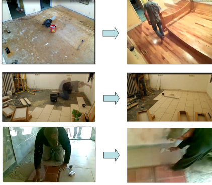
Figure 17: Example of temporal trends in event E019, "Installing Flooring." Many videos start off with a bare floor followed by a floor that has been further finished. However, some do not have a clear direction from the camera angle given.
