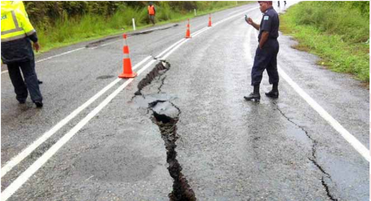
Slip at Naibore Hill, Kings Road after heavy rain, February 2014 Source: Ministry of Information, Fiji News Summary (Minfo News [news@info.gov.fj])
