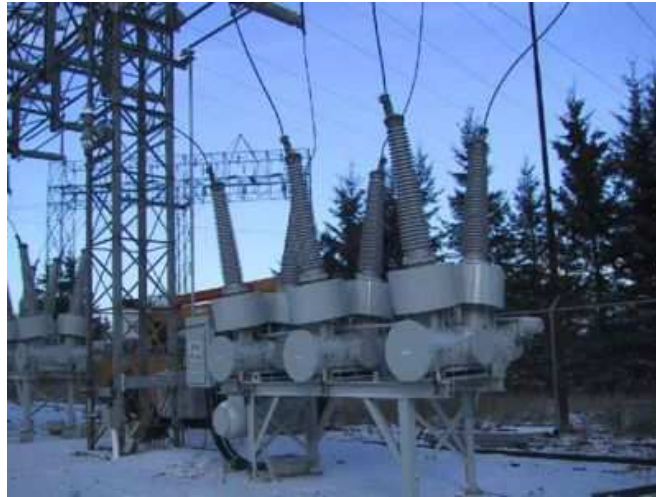
Figure 2.3: Dead tank circuit-breaker (Source: Manitoba, Canada)
