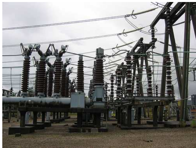
Figure 2.7: Air-blast circuit-breaker (Source: Strathaven substation, Lanarkshire, UK)
