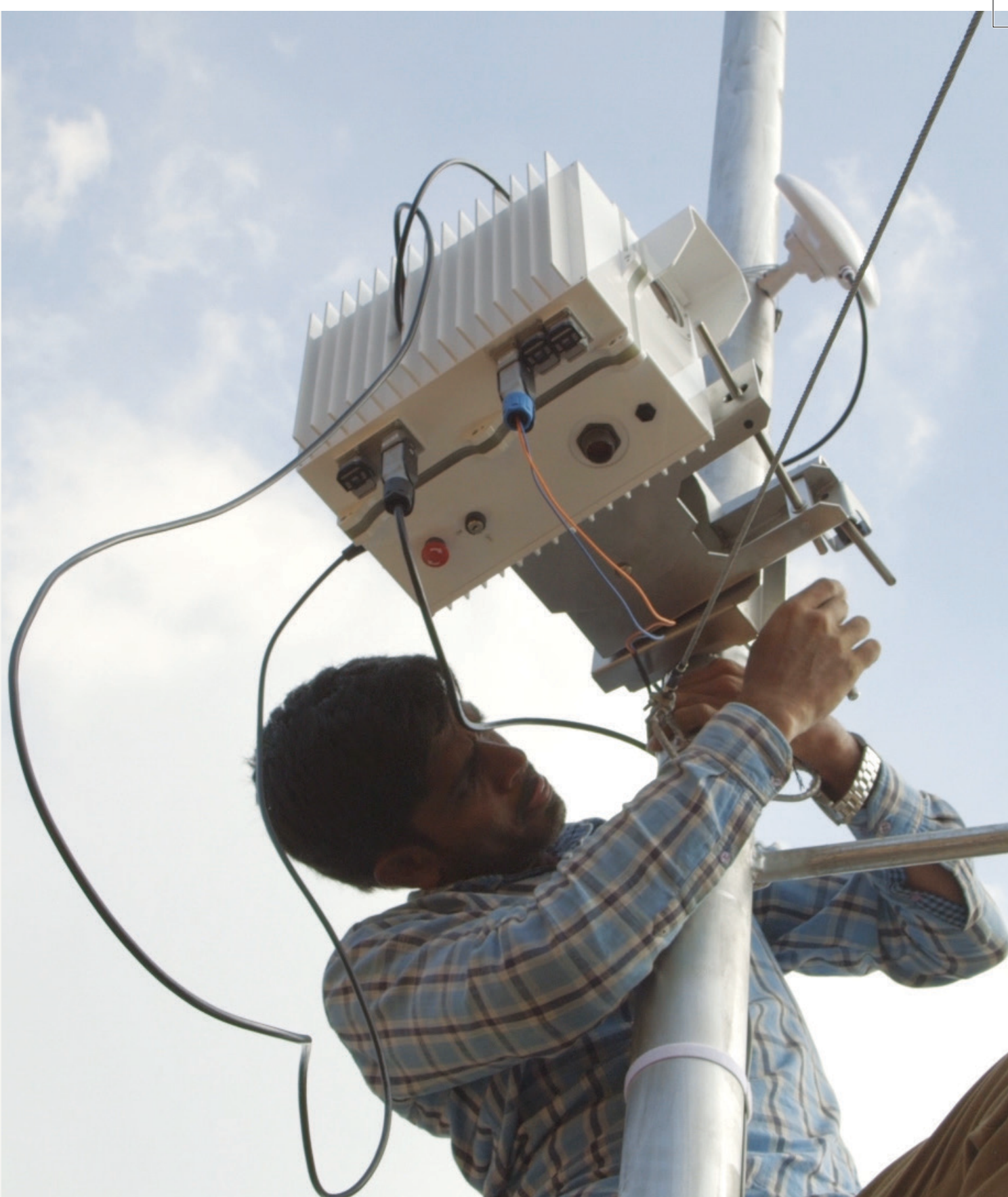
^ A free space optical communications [FSOC] unit is installed for a broadband connectivity test in the Indian state of Andhra Pradesh
