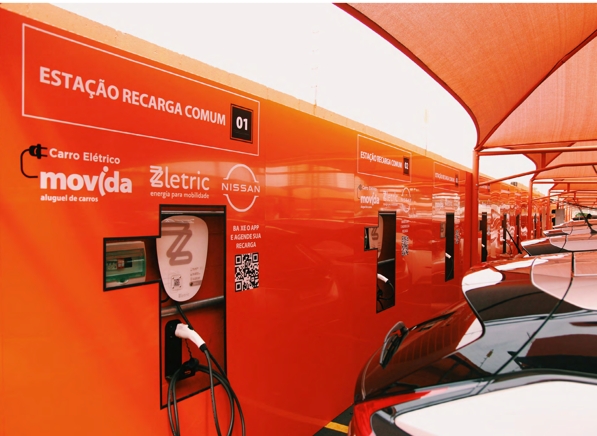
Electric Vehicle Charging Station | Moved
