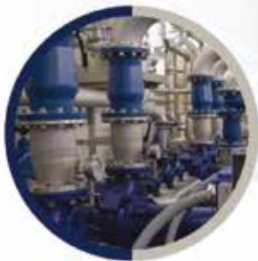
Industrial Pump Control
