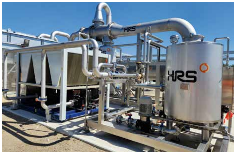
The HRS BDS at Melbourne Water's Eastern Treatment Plant incorporated some complex design elements.
