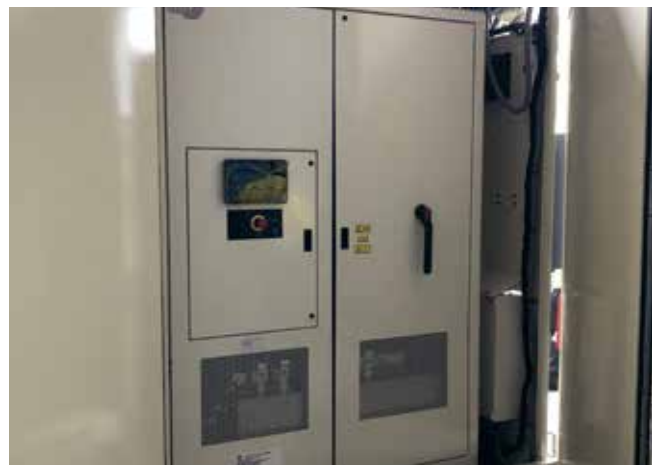
The RUC team chose Rockwell Automation to supply the regenerative variable speed drives for the regenerative energy storage solution.
