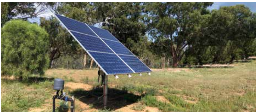
An automated solar array that delivers the right amount of water at the time it is needed, with PLC control allowing this to be remotely adjusted according to conditions.
