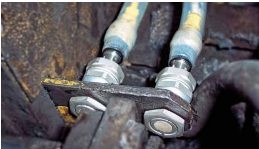
Figure 3: Silicone wrap protects the cable and connector.
