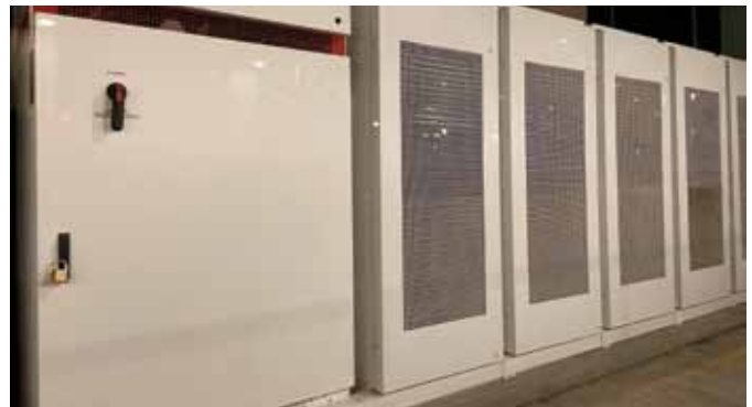
When charging, UQ's battery bank is lit green. When discharging, it lights up blue. Image courtesy The University of Queensland.
