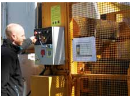
SCG Venue Manager Alex de Graaf operates the venue's co-mingled compacter.
